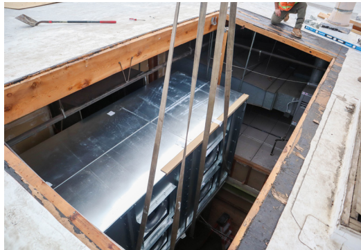
A section of the new Trane Split System 80-Ton Condenser 44,000 CFM Air Handling Unit being lifted via crane through the roof opening.
